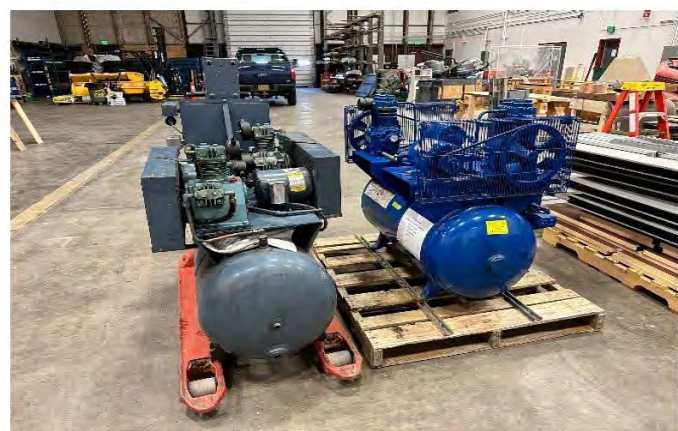
Old Compressor (left)
